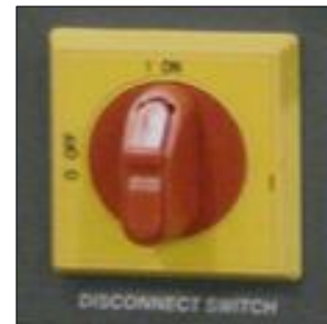
Figure 21. Main Disconnect Switch.
