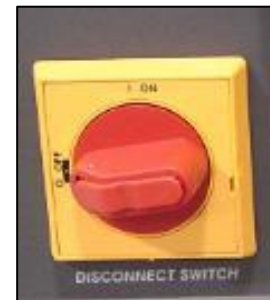
Figure 1. Main Disconnect Switch.
