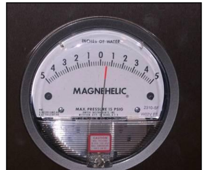
Figure 6. Magnehelic Pressure Gauge Measures Pressure in Front of the HEPA Filter.
